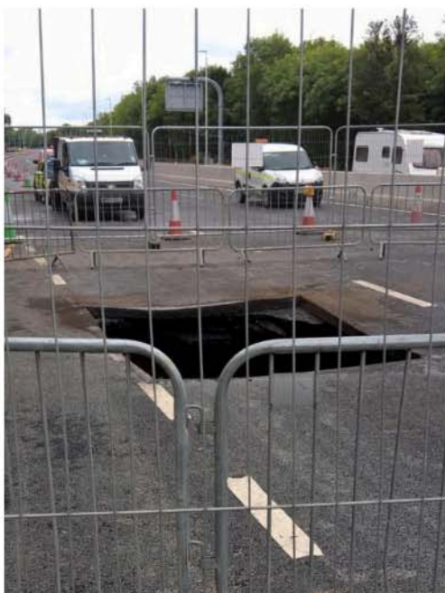
Figure 1 Mineshaft collapse in Lane 1 of A1M in 2016 (Source: GDMS Geotechnical Event ID 45)
